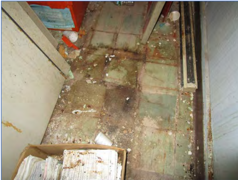
Photograph 7 – Water damaged 9” x 9” asbestos vinyl floor tiles and black mastic.
