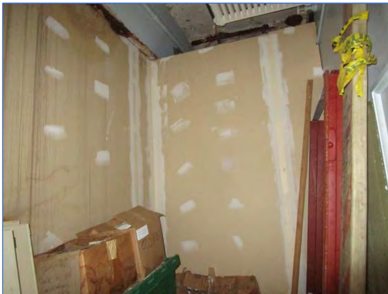
Photograph 8 – Water damaged drywall in the paper/file storage room.
