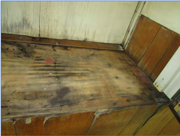
Photograph 5 – Water damaged and moldy wood associated with sealed windows in break room area.
