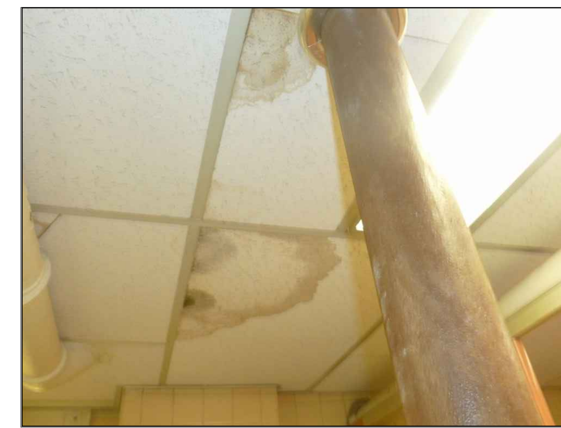
2 CEILING TILE DAMAGE
