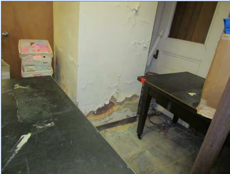
Photograph 3 – View of Water damaged Asbestos containing plaster.
