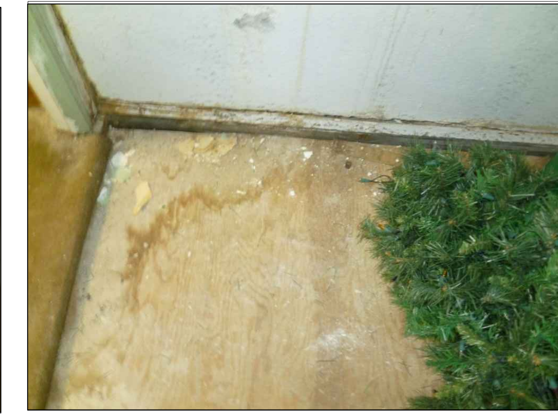
3 FLOOR CARPETING DAMAGE
