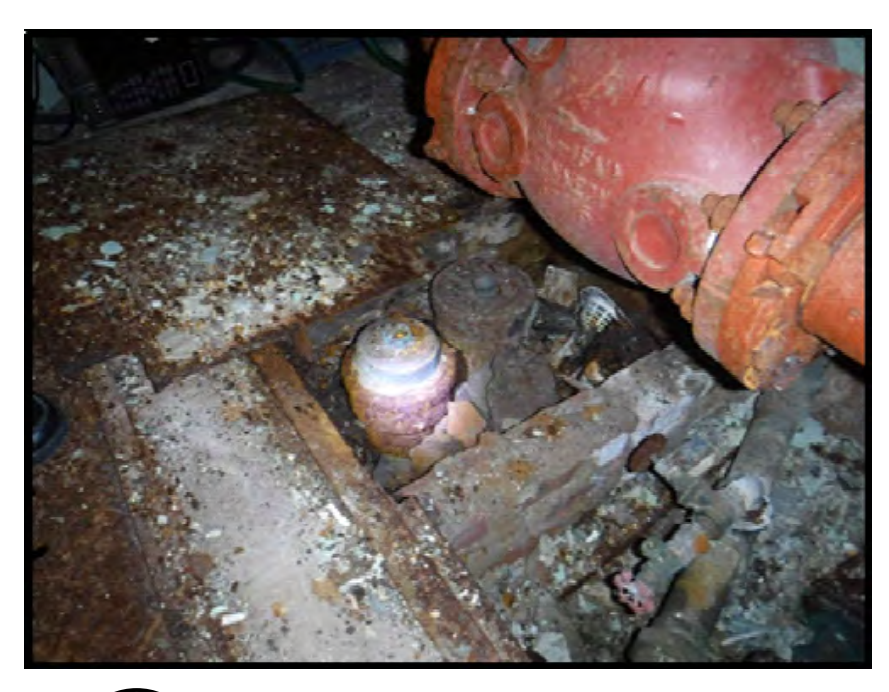
2 EXISTING HOUSE TRAP
