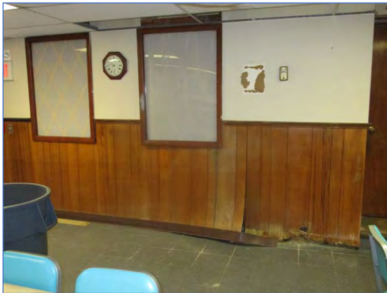
Photograph 2 –View of basement break room with poorly sealed windows to the outside and water damaged wood paneling.
