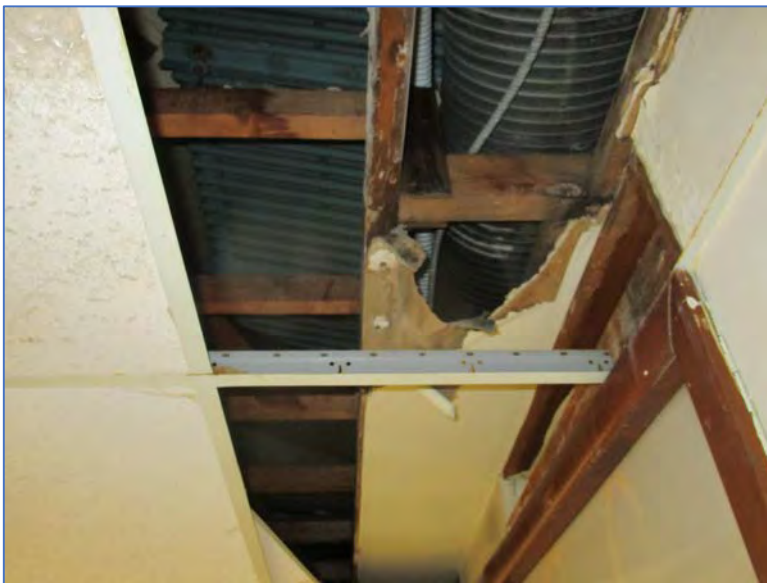
Photograph 6 – View water damaged drywall ceiling above drop ceiling tiles in the break room area.
