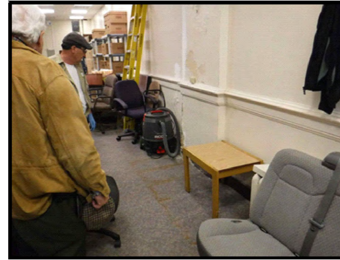
1 FLOOR AND WALL DAMAGE
