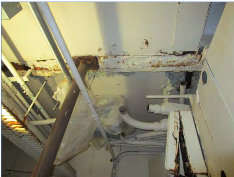
Photograph 4 – View above storage closet and damaged plaster. This area has experienced leaks for several years per maintenance staff.
